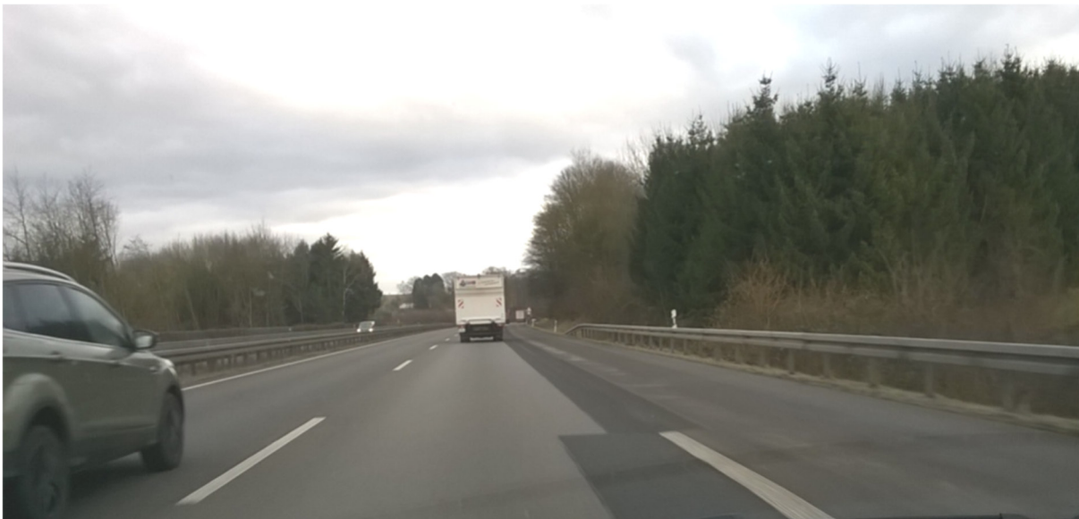
Fig. 5 Segment with missing road markings on one side of the lane
