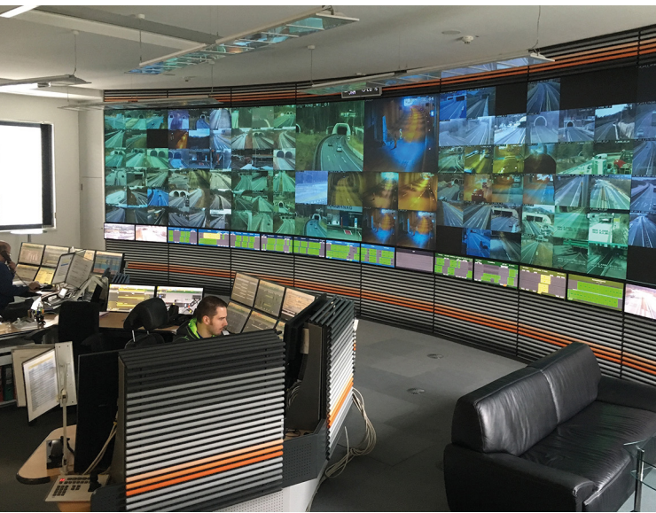
Tunnel Control Centre (Photo: DÜRR Group GmbH)
